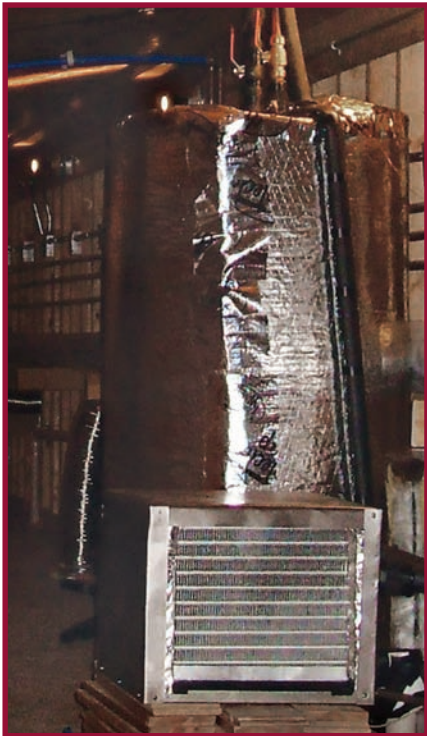
Photo 3: Heat pump water heater installed in Equinox House with additional tank insulation.
