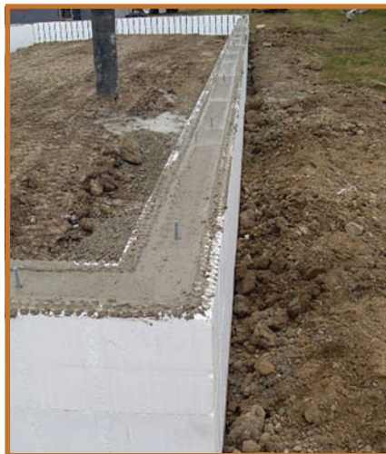
Photo 3: Concrete poured in ICF foundation wall. The exterior ground is graded to 8 in. (200 mm) below the top of the ICF foundation wall.
