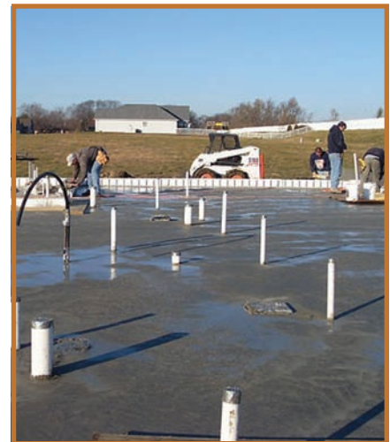
Photo 4: Floor slab and exterior grade are 8 in. (200 mm) below the top of the ICF foundation wall to provide barrier free entrances into Equinox.
