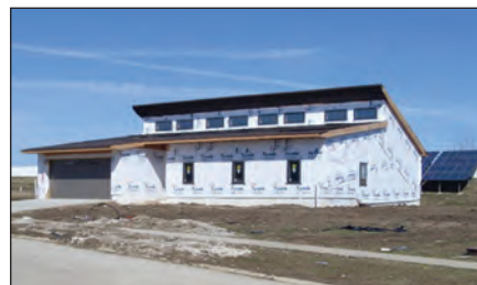
Photo 3: Completion of the building shell with windows, eaves, and house wrap. The photo was taken on the spring equinox (March 22). Note the overhang shadows at the top edge of the windows when exclusion of direct solar radiation begins.
