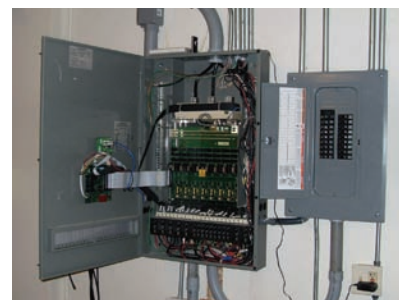
Photo 2a (top) and 2b (bottom): Computer controlled electric circuit breaker panel in Equinox House. Note the cell phone modem on top of the unit for Internet communication and the adjacent subpanel.
