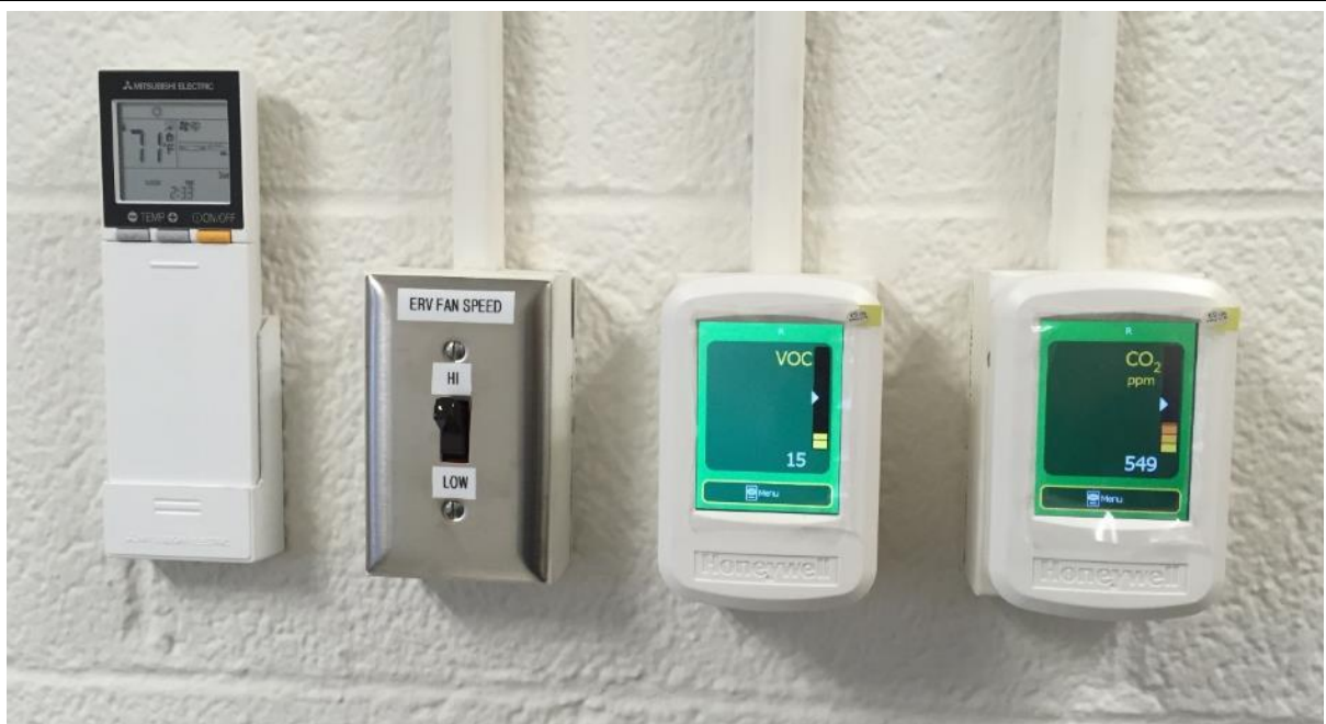
Photo 3 Local comfort control and air quality control in the MechSE UG Advising office. Both VOCs (Volatile Organic Compounds) and carbon dioxide concentration must be measured and fresh air ventilation automatically activated when either exceeds occupant selected thresholds. Local comfort is equally important with simple control of heating and cooling.
