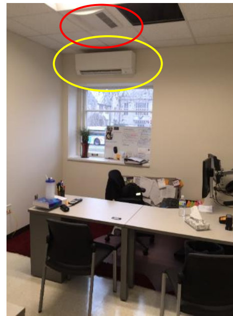
Photo 2 Interior view of MechSE UG Advising office with local comfort control (high performance, low temperature mini-split heat pump) and fresh air ventilation. The yellow circle identifies the quiet, high efficiency, cold temperature mini-split heat pump unit. These units are standard in commercial and institutional buildings outside of North America. The red circle shows the fresh air vent connected to the local energy recovery unit hidden above the office ceiling. Local fresh air allows each office and classroom to be efficiently managed, increasing occupant productivity and satisfaction, while minimizing the spread of illness to the building's occupants.
