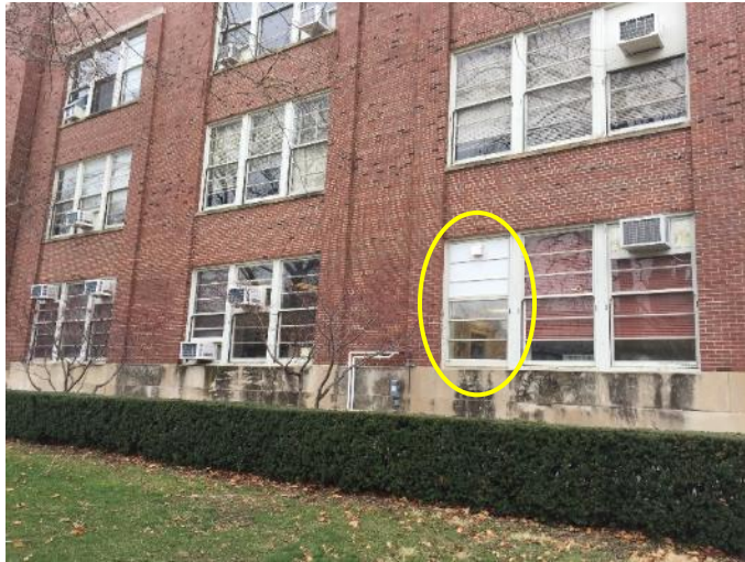
Photo 1 UG Advising office with local fresh air vent and reduced window area. Yellow oval shows UG Advising Office with upper window replaced with insulated panel and local fresh air supply vent. Note window shades drawn in the excessively windowed offices and classrooms. Efficient, localized comfort conditioning such as the low temperature mini-split heat pump in the UG Advising Office can replace unsightly window AC units at a cost much lower and an efficiency much higher (SEER 30) than central conditioning systems, while keeping building occupants healthier and more productive than centralized ventilation systems.
