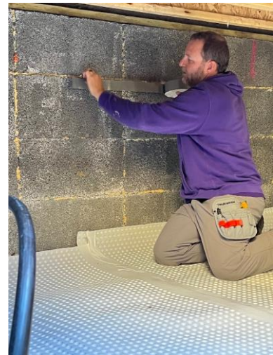
Figure 3 Matt Blomquist is instructing his students on installing double stick mastic for sealing crawl space poly film to ICCF foundation wall.
