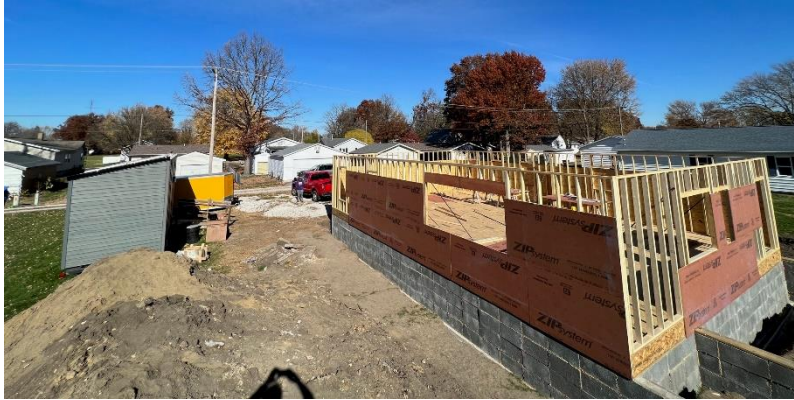
Figure 2 November 15, 2023 photo of THS PGH work site. Follow Matt Blomquist's build_learn_teach instagram site to watch the progress as it happens. Solar power from the work shed powers house construction activities!
