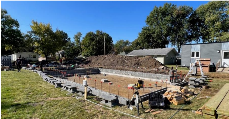
Figure 1 October 10, 2023 installation of ICCF (Insulated Composite Concrete Form) walls by Taylorville High School students.
