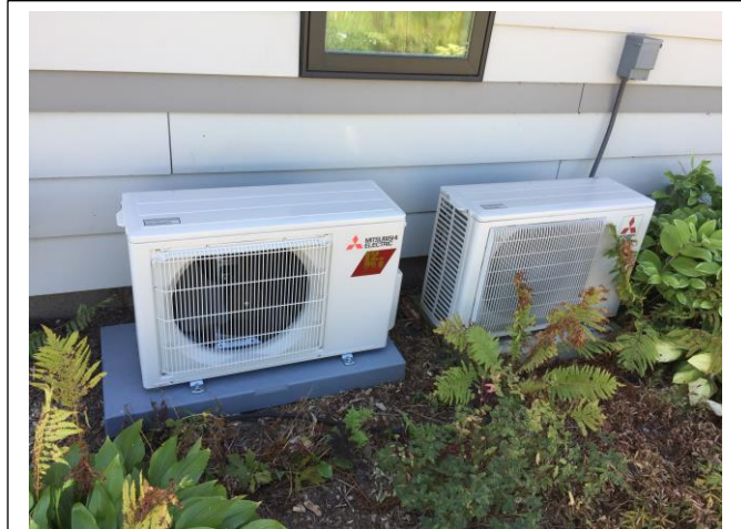
Figure 2 A ¾ ton mini-split has been added to the original 1 ton mini-split in Equinox House. The new unit has been installed to demonstrate the CERV2's ability to control distributed mini-splits with our CERV-IR (CERV-Infrared) technology. Other than minor differences in looks with an 8 year age difference, the two minis are identical. The two minis give us an efficiency boost over the single mini in summer and winter!
