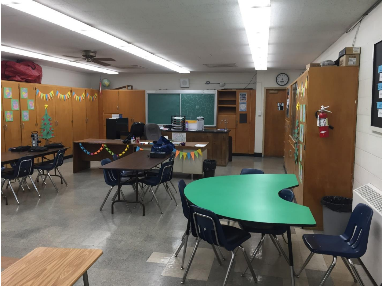
Figure 6 Conversion of incandescent lighting to energy efficient LED lighting in older schools, such as MMJH, provides electrical panel capacity for CERV-1000 operation. Room 111's original incandescent lights required three 20amp breakers. Each row of LED lights draws only 2amps, allowing all classroom lights to be combined on a single 20amp breaker, making room for the CERV-1000 40amp, 2-pole breaker.
