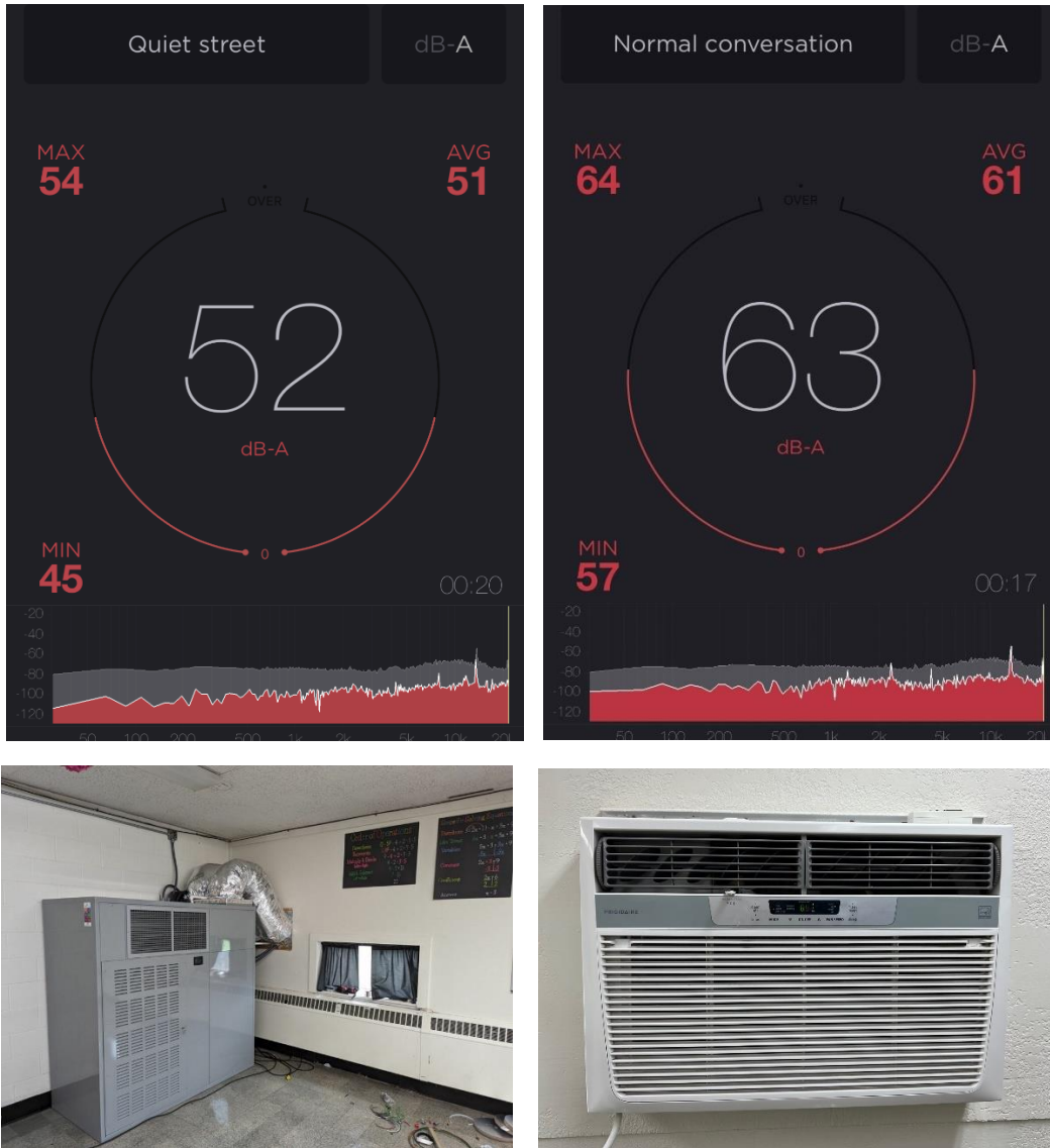
Figure 9 Blowing 1000cfm quietly into a classroom, restaurant, house of worship or other high occupant density space requires a lot of considerations to keep noise low. Sound readings shown are from identical, adjacent classrooms with the sound meter placed at the same relative location from the CERV-1000 and window AC unit. The CERV-1000, with ventilation fan on high, is more than 10 times quieter than the window AC unit.
