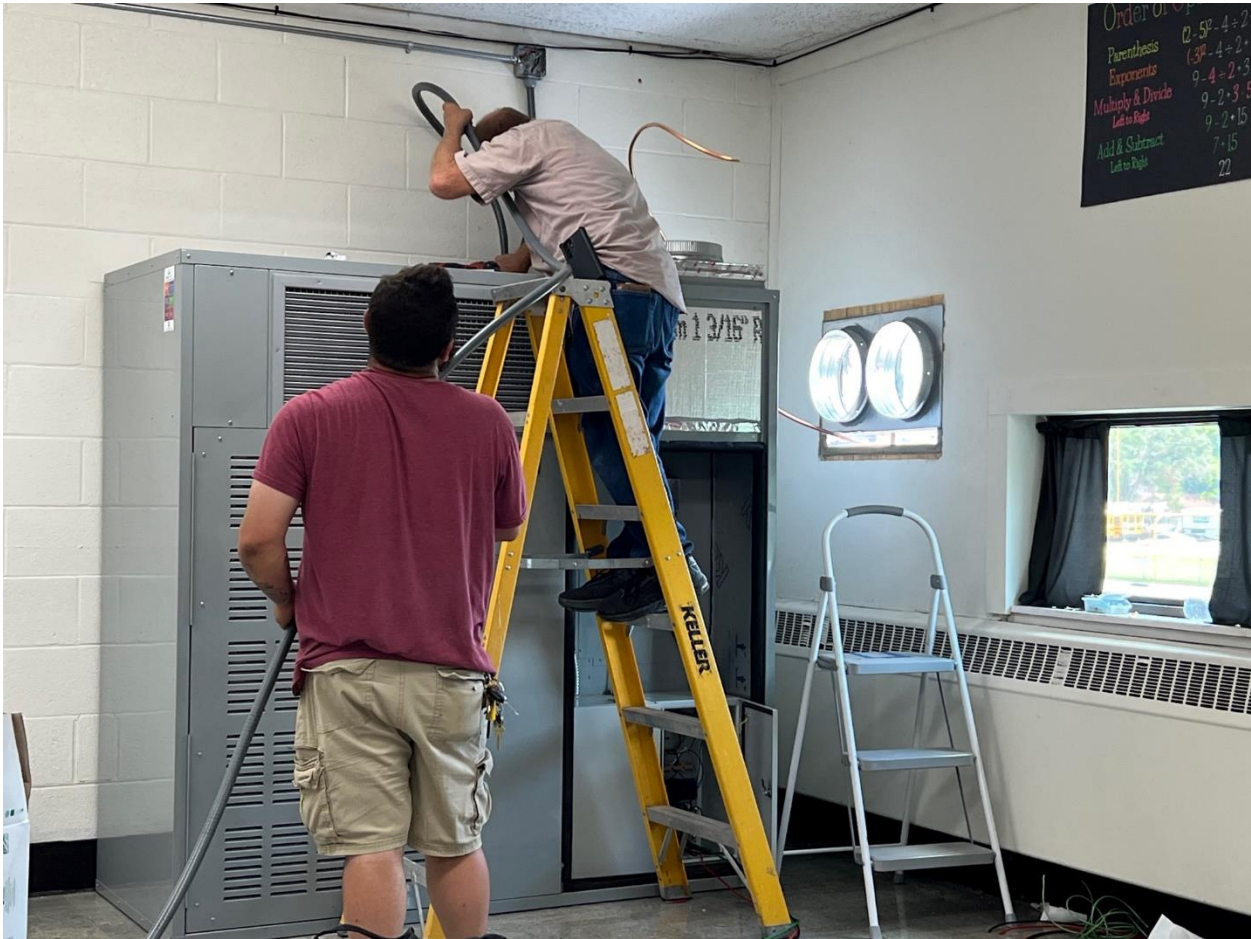
Figure 5 Georgetown-Ridge Farm School District's Facilities Director and one of his maintenance staff install CERV-1000 power wiring. The unit requires 8 gauge wire and a 40amp (240VAC) breaker, which is often available in schools that have substituted LED lighting for incandescent lighting.
