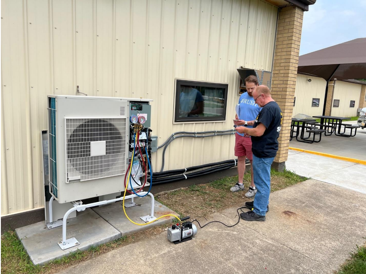
Figure 7 G-RF Facilities Director Reuben and Build Equinox co-owner and Vice President, Alex Long, are checking out CERV-ICE on their phones, our online monitoring and control dashboard. Reuben is looking forward to increased maintenance efficiency of CERV-1000 units. He spends significant time moving among the school district's three campuses (elementary, junior high and high schools). With CERV-ICE, Reuben can conveniently check classroom air quality, comfort, and operation of every CERV-1000 unit in the school district.
