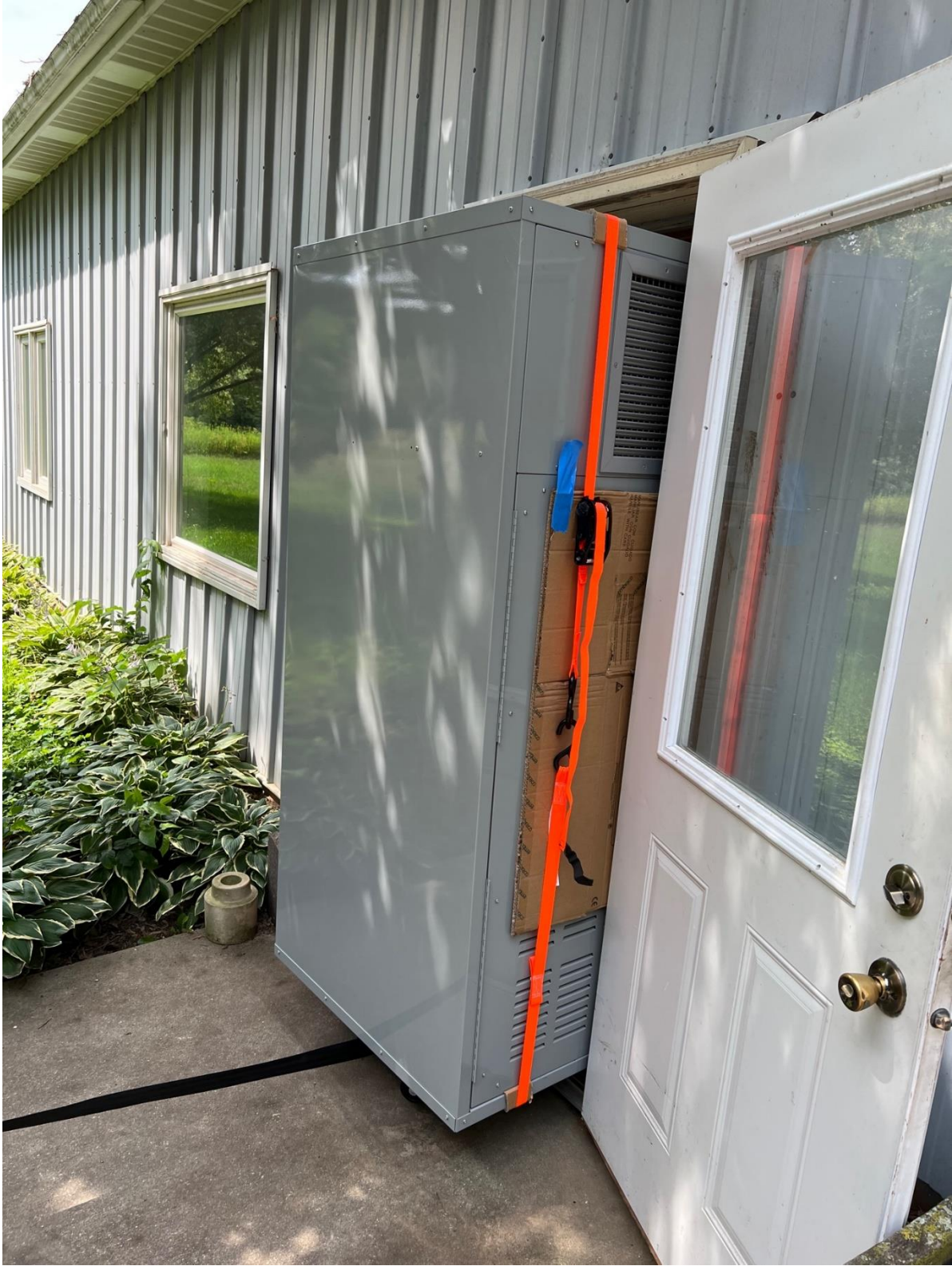
Figure 4 CERV-1000 units are designed to fit through standard 36" doorways. CERV-1000 Unit#1 is moving through Build Equinox's business facility doorway on its way to MMJH School Classroom 111.
