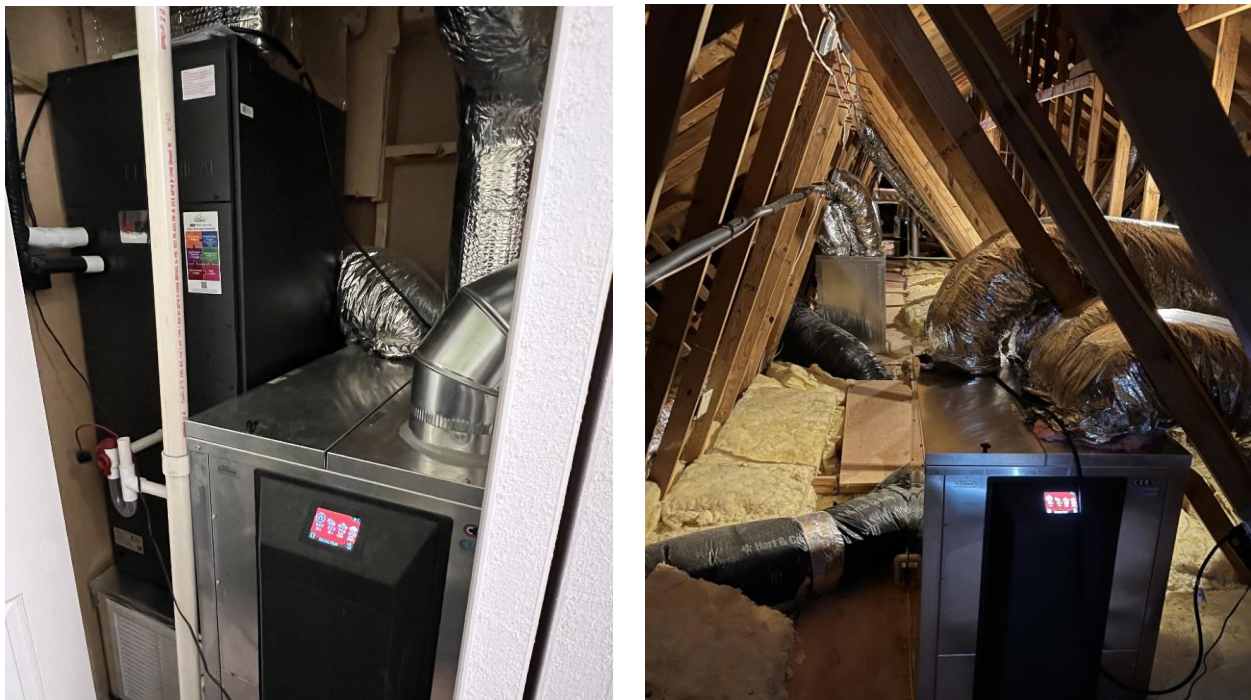
Figure 2 Five CERV2 units were integrated into existing ductwork for distribution of fresh air throughout the building. The left photo shows a heat pump air handler with CERV2 located in a mechanical closet on the first floor. Three CERV2 units were paired with ductwork from three inactive propane furnace units in the attic.
