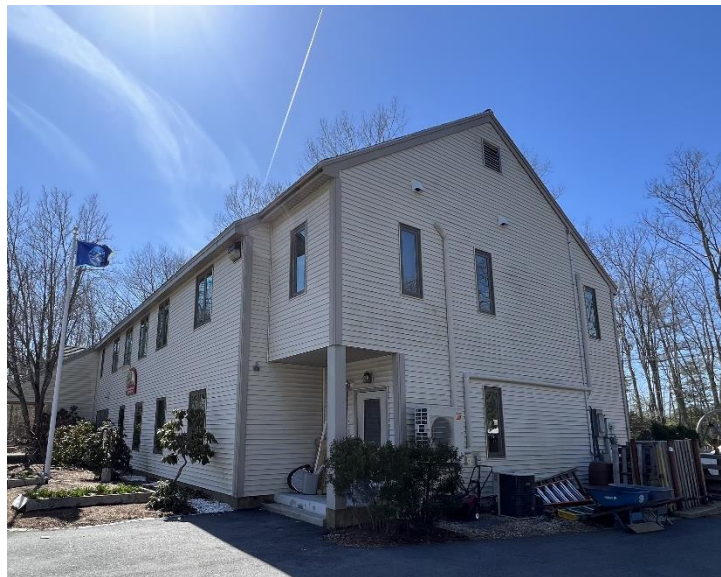
Figure 1 Heat pump outdoor units (ODUs) located on each end of the BMFS building.
